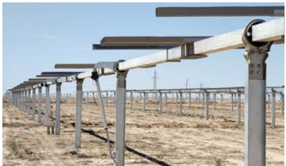
Trina Tracker installed in Habei, China, 400 MW
